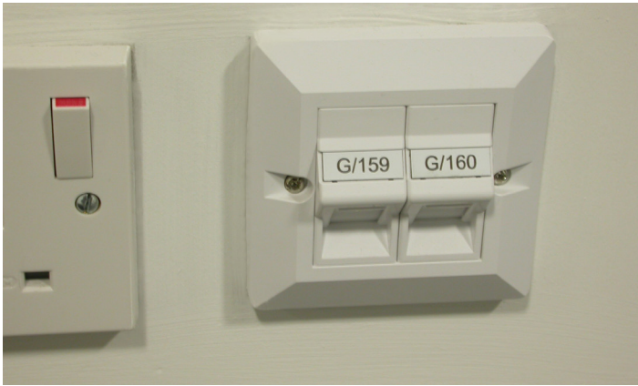
Angled wall outlets with Traffolyte labelling
