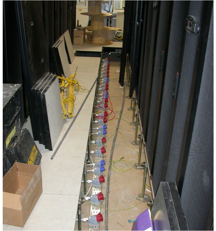
Data centre nearing completion before the servers are moved in.
