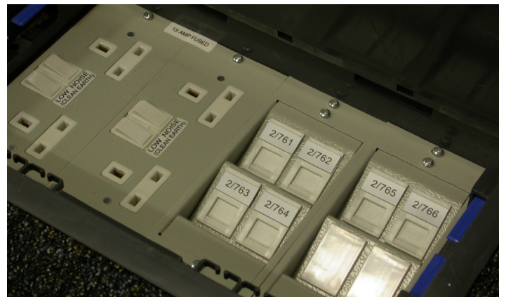
Floor box in one of the meeting rooms
