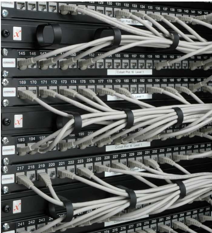
Net10G patch panels and cable management
