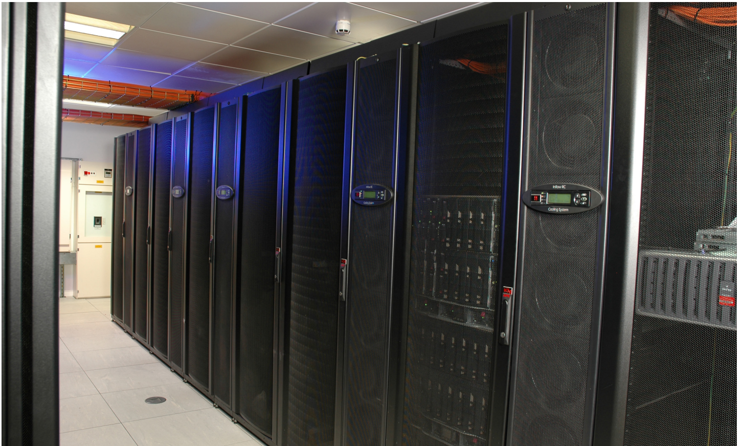
The completed cold aisle with just some of the shielded Net10G LSZH data cable in tray overhead
